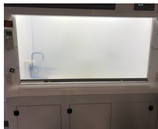
Visibility through sash impaired due to etching from HF acid use. Can you see the white bucket?
